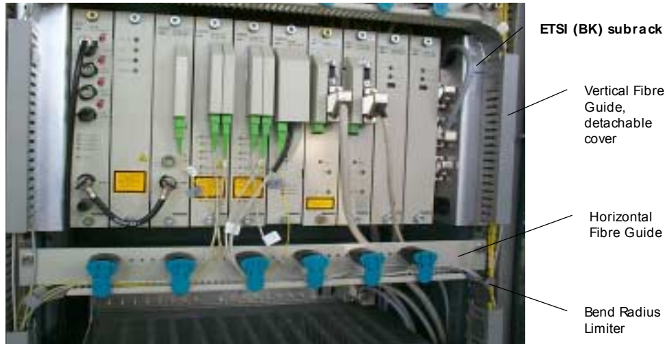
Figure 4-3: Fibre Optic Cabling at BK-subrack
